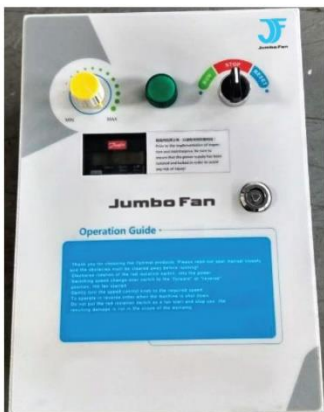
Danfoss Controller box
